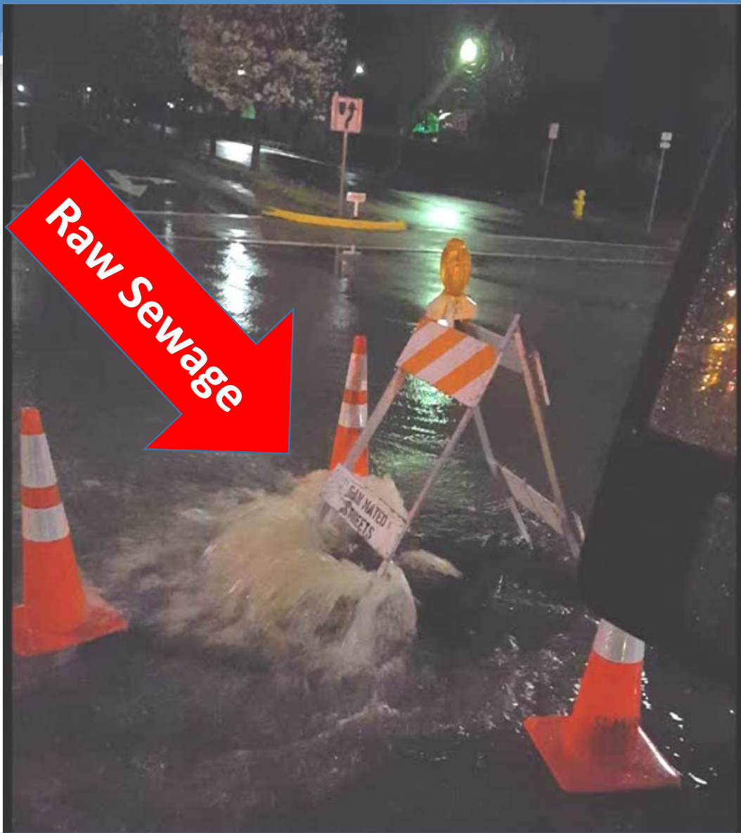
Sanitary Sewer Overflow (SSO) at Saratoga Dr & Delaware St
