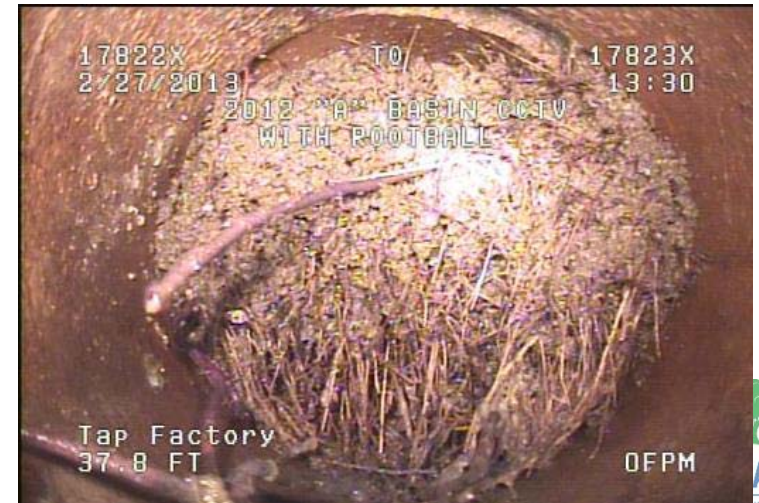
Root Intrusion into Pipe
