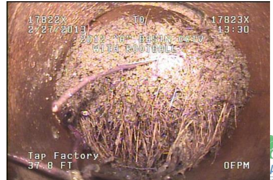
Root Intrusion into Pipe
