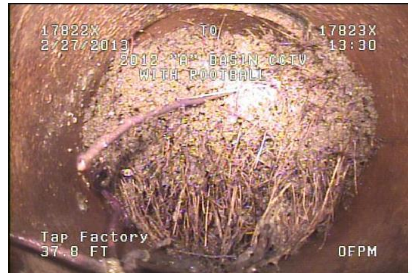
Tree Roots Blocking Pipe
