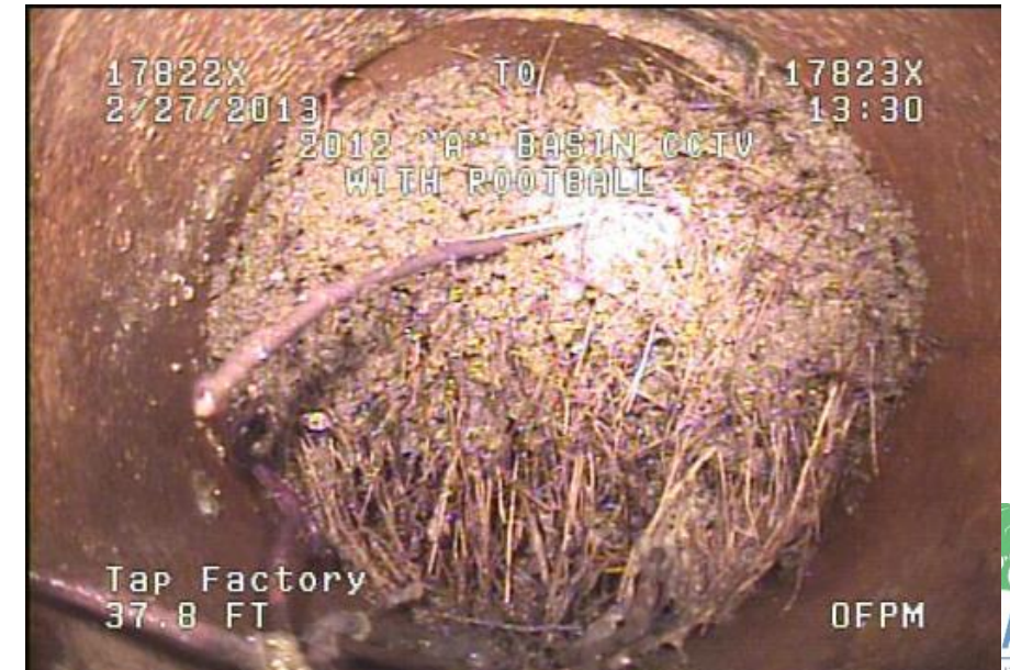
Root Intrusion into Pipe
