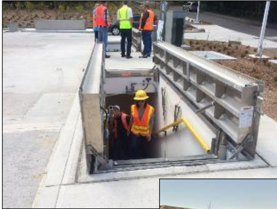
Example of ground-level air-tight vault access hatch (typically closed)
