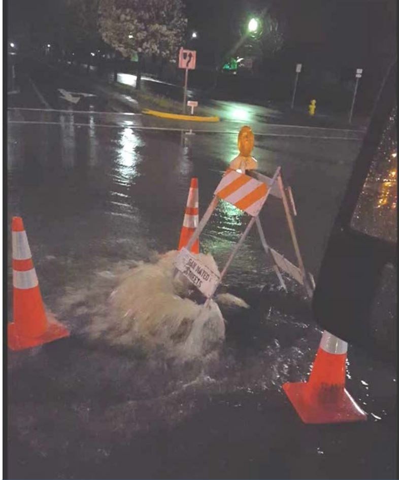
Sanitary Sewer Overflow (SSO)
